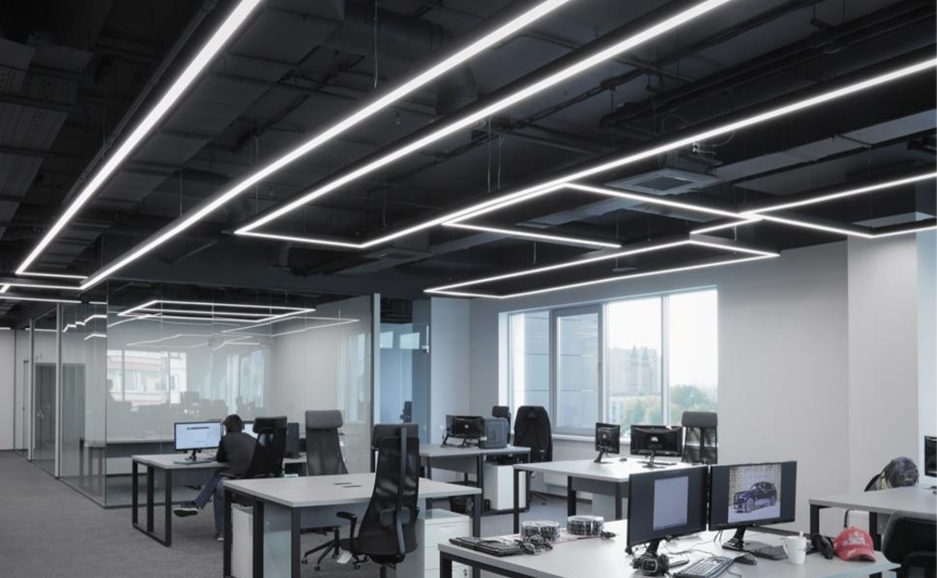
IT company "Katyusha IT" | Installed: PROFILE LED, SLIM LED, SOL P LED
