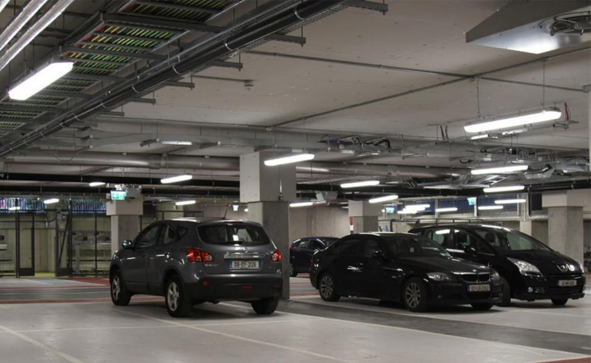
Exchange building office | Installed: PILOT DL LED, SAFARI DL LED, ARCTIC range
